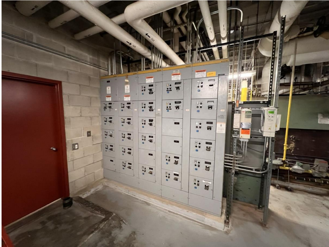
Typical electrical equipment to be modified
