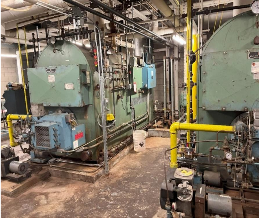
Boilers to be replaced
